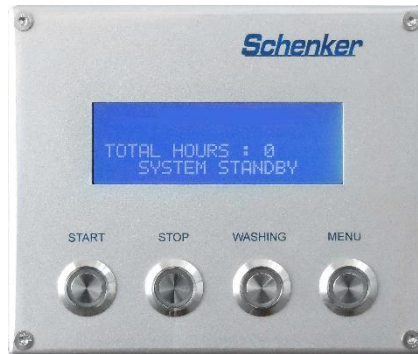
Remote control panel Fig. 5.1
